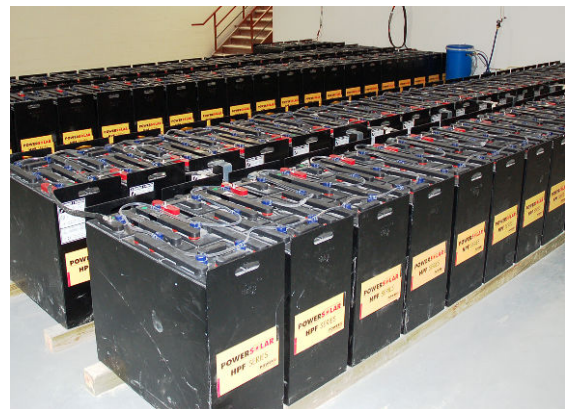
Figure 2-1. A battery array providing 60KW at 480VDC as backup for a corporate data center. (Photo by permission of Hybridyne Power Systems, Canada, Inc., and the Hybridyne group of companies. Copyright by Hybridyne, an internationally registered trademark of Hybridyne Power Systems Canada Inc. No right of further reproduction unless specifically granted by Hybridyne.)
